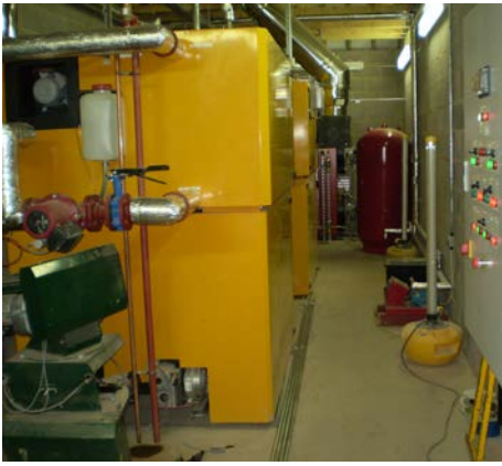
KWB TDS Powerfire boilers in plant room
