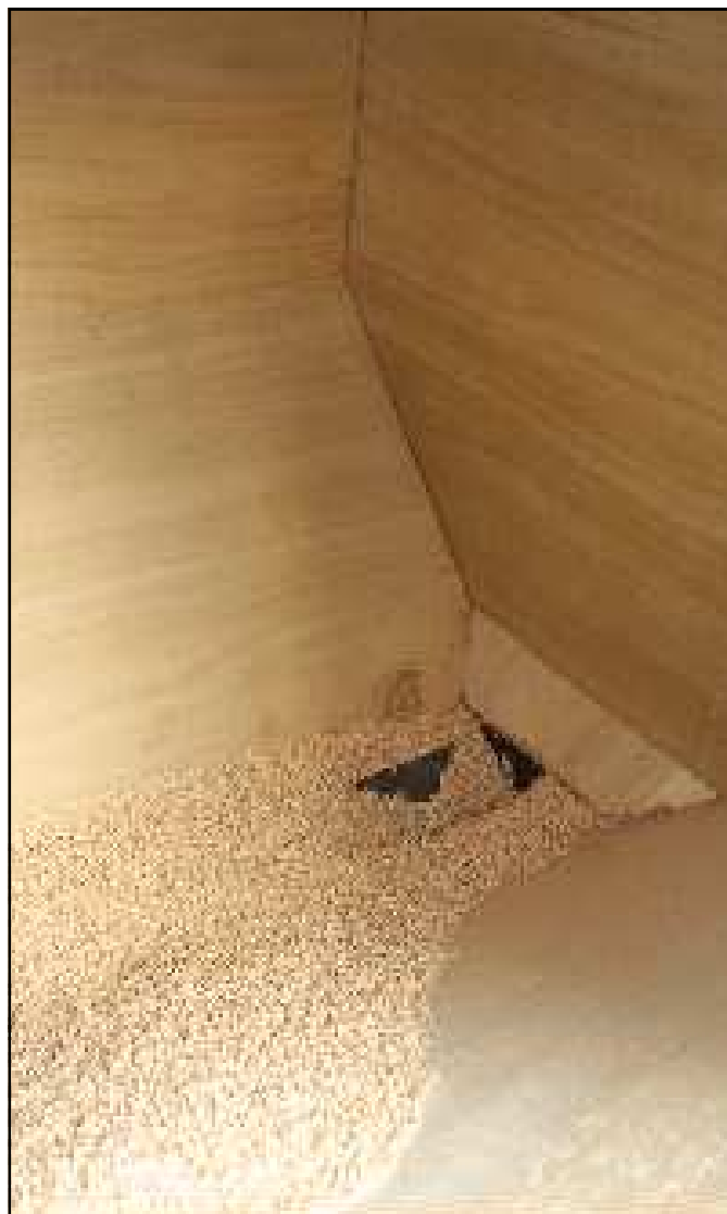
Right - Inside pellet fuel store, built on site, with V shaped sides running into feed extraction
