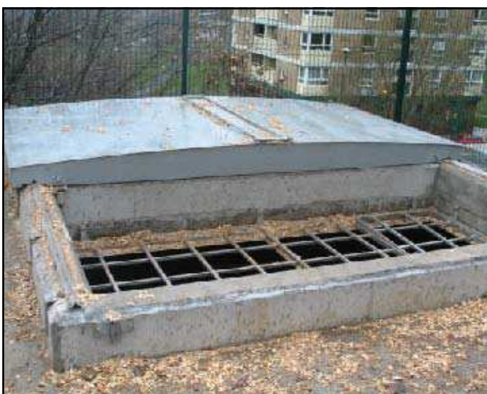
Top left; Boiler room (behind) & fuel reception bunker Middle left; Lorry access to fuel reception bunker Bottom left; Manual push-back bunker lid awaiting a fuel delivery
