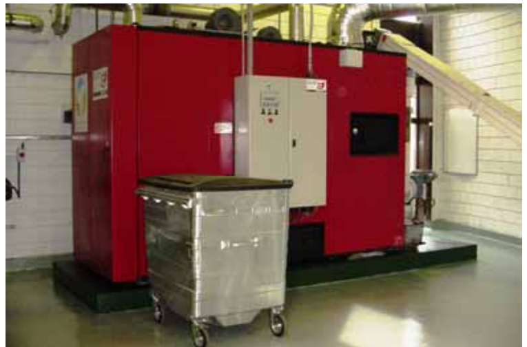
Compact 700 kW woodfuelled boiler installed at Worcestershire County Hall
