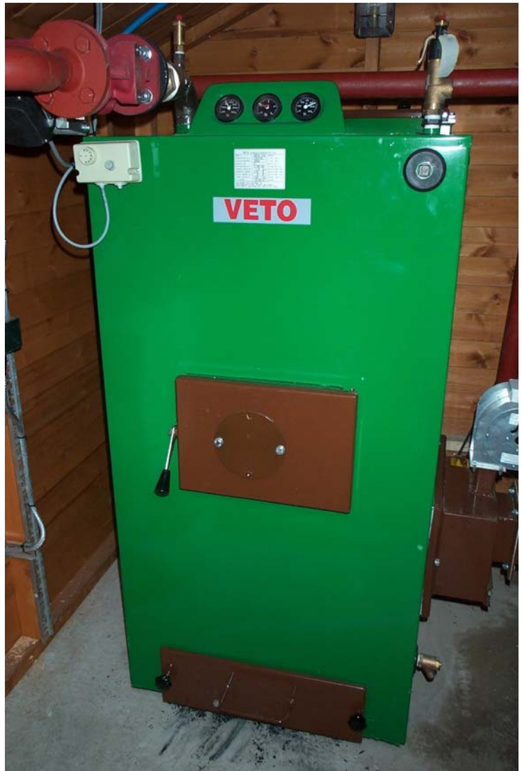
Veto 120 kW stoker-boiler (burner head on the right)
