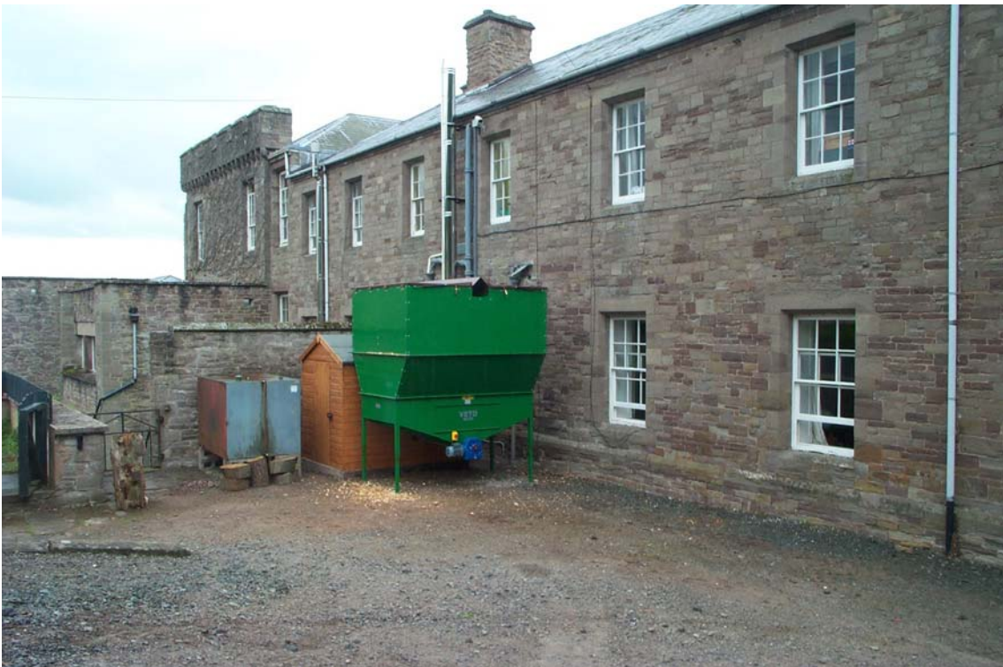
The woodfuel hopper and boiler house
