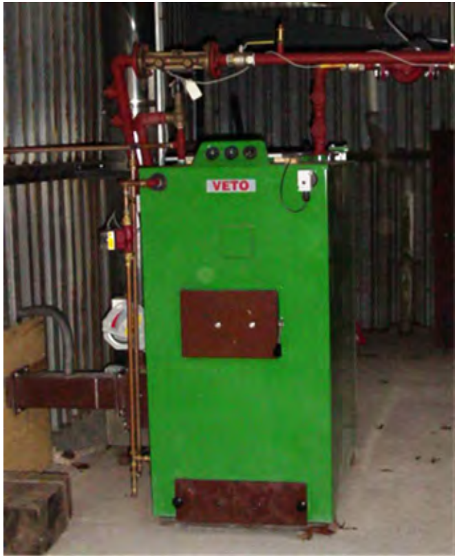
Veto 100 kW stoker-boiler, fuel feed from left
