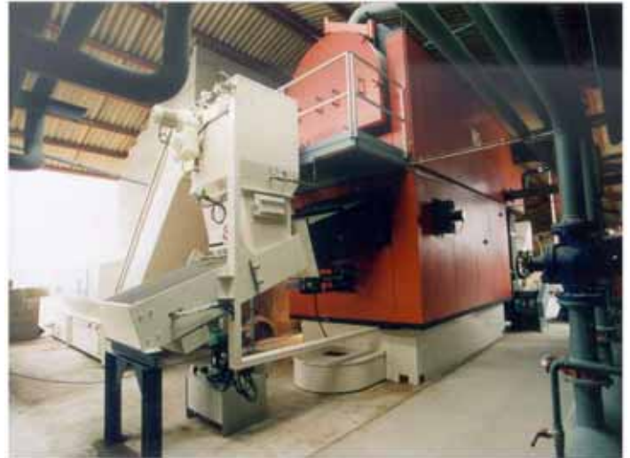
A Compact C250 DHP 2,500 kW wet-wood boiler with ram stoker
