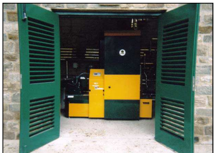
KWB USV D 100 kW automatic woodchip boiler, fuel feed from left, ash bin on right
