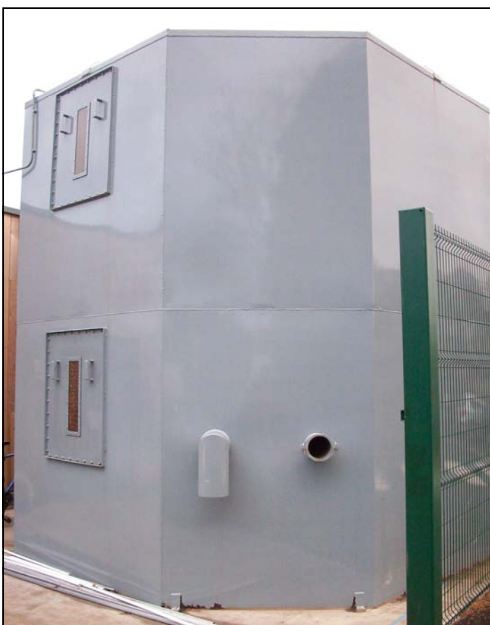
Above; Boiler room and fuel store Below; Close up of steel fuel store, showing the blown fuel inlet and air outlet pipes
