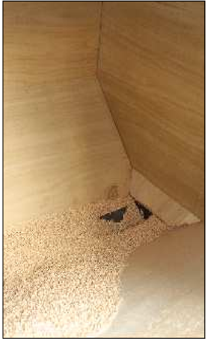
Right - Inside pellet fuel store, built on site, with V shaped sides running into feed extraction
