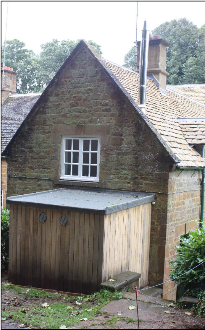
Left - Purpose built pellet store, showing storz 'A' pellet connections.
