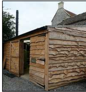
70kW Log boiler with solar thermal panels Farm in Somerset. Eco Engineering
